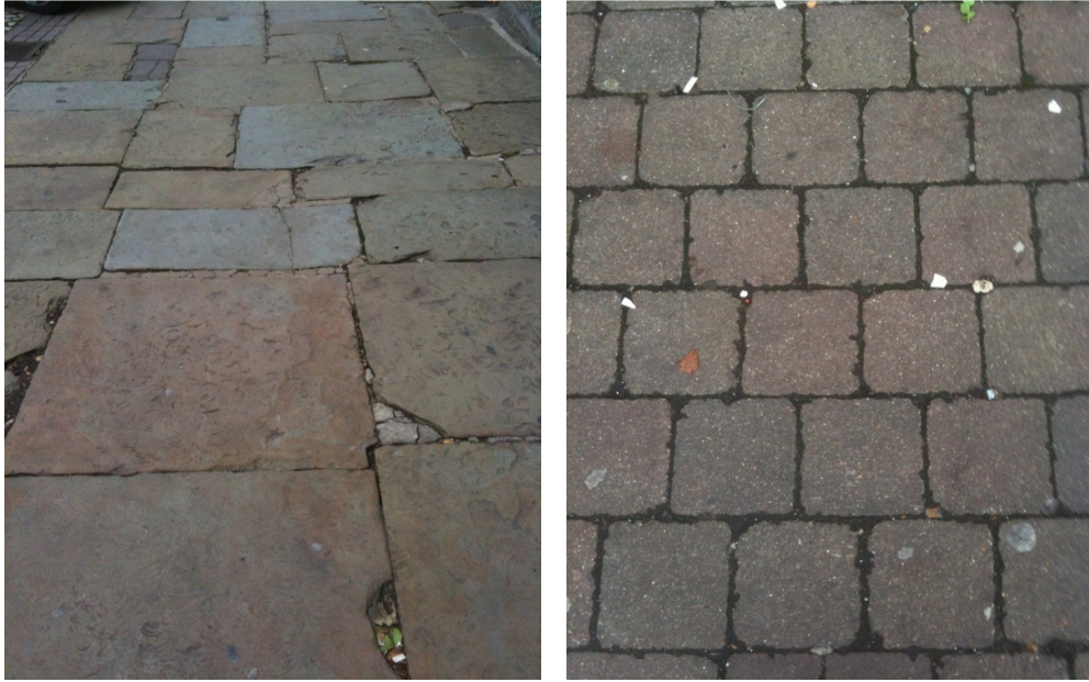
Figure 2: Paving styles around the public realm, varying from high quality, but damaged natural stones, to more pragmatic manufactured blocks.
